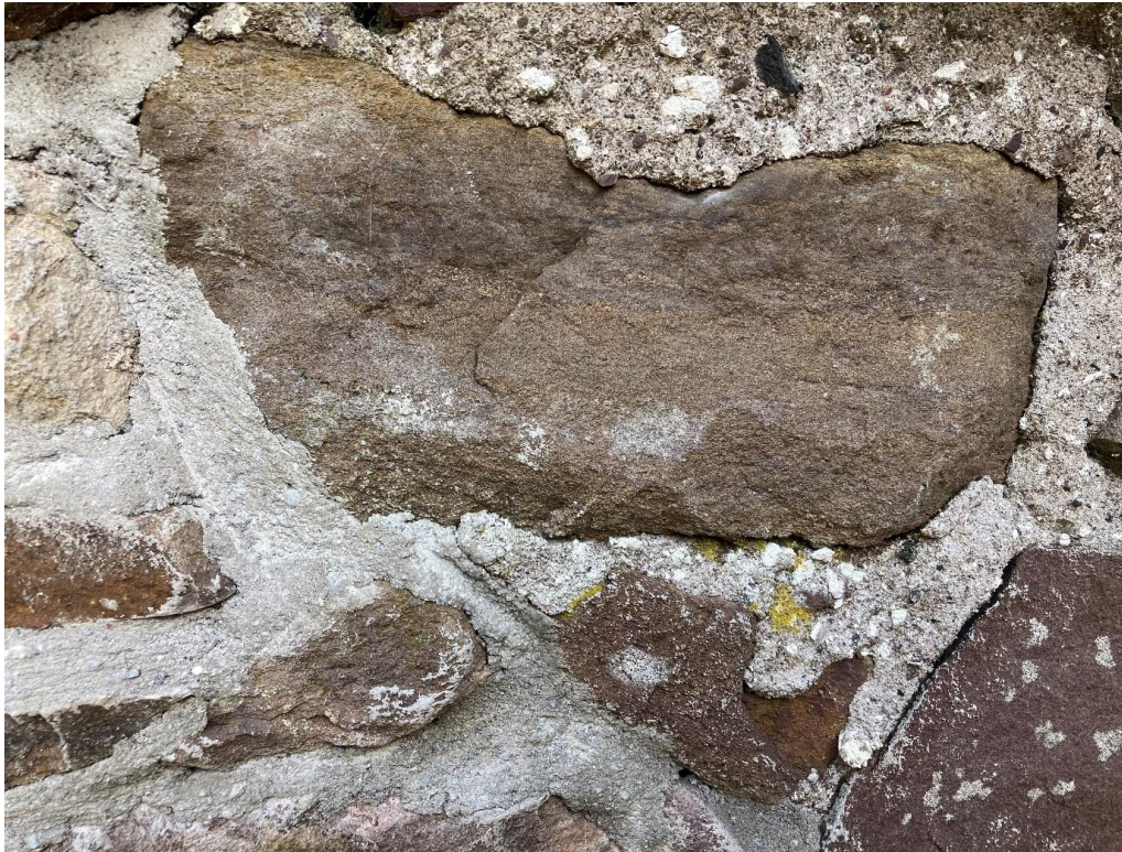
Plate 8: Note the difference between the unsatisfactory new pointing on the left and the original mortar to the right. There is no coarse aggregate in the new mortar, resulting in a loss of the character of this structure.
