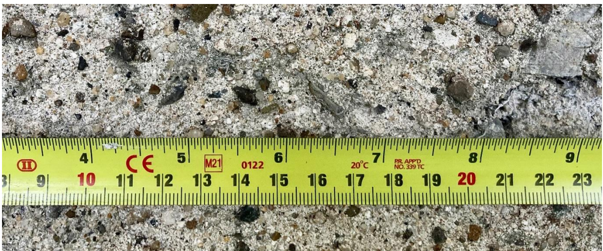
Plate 2: Size of stones in the mortar from Plate 1.
