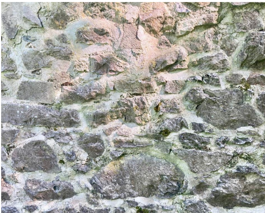
Plate 9: This is a poorly repointed wall; no pinnings have been used in the mortar and there is no exposed aggregate. The character of the structure has been lost.
